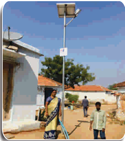
SPV based LED Street Lighting System
