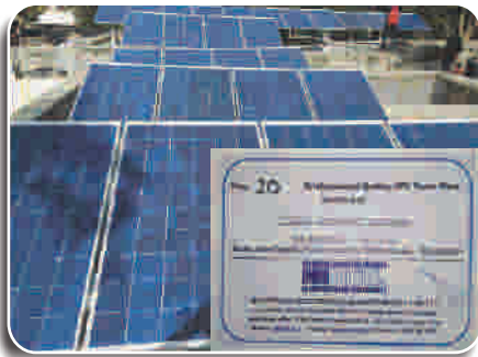
SPV Grid-connected RTS at building of Forest Department, Rajasthan
